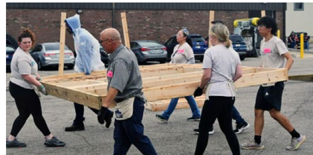
› Habitat for Humanity Arcwood volunteers spent the day building a new home in the community with Greater Indy Habitat for Humanity in what has become a yearly event.
